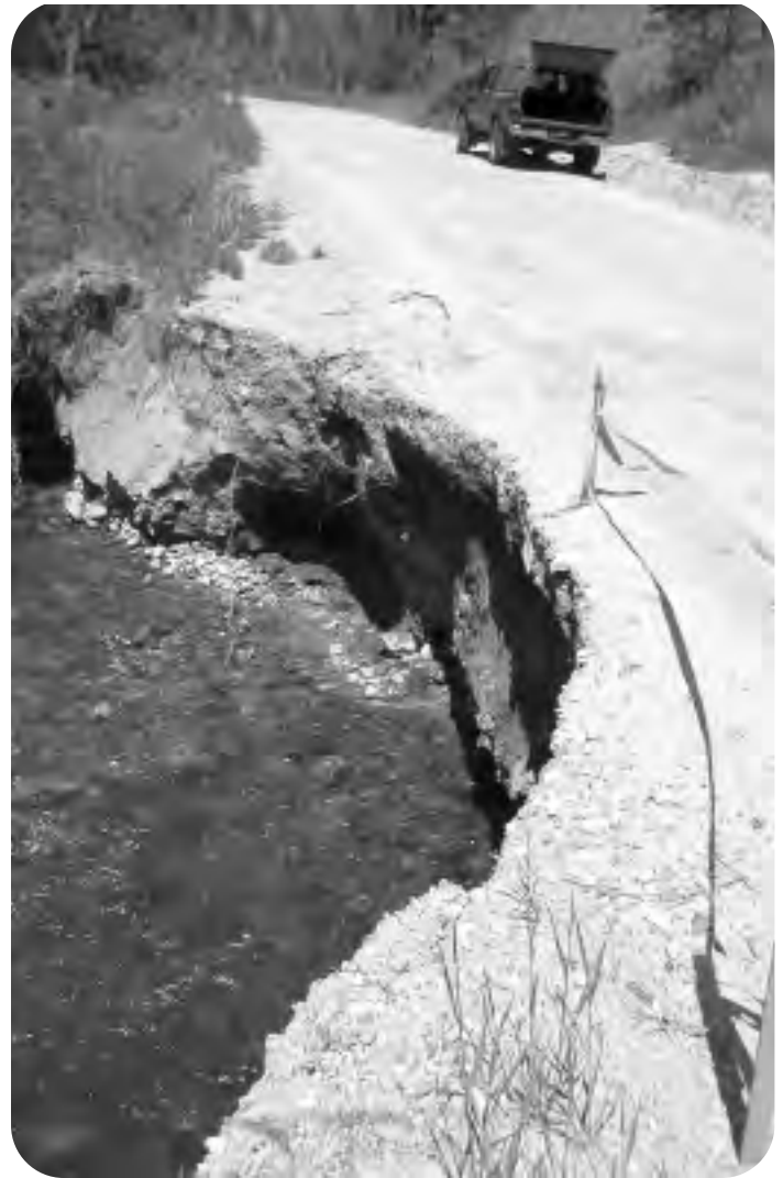
There are real, on-the-ground consequences associated with the Forest Service's failure to complete promised road and water restoration work as part of the "Burned Area Recovery Plan." With over $16 million slated for critical non-logging restoration and rehabilitation activities taken away from the Bitterroot Burned Area Recovery project by Chief Bosworth to pay for firefighting costs of the 2002 fire season, nearly 75% of the promised restoration work remains undone. Photo by Matthew Koehler.
