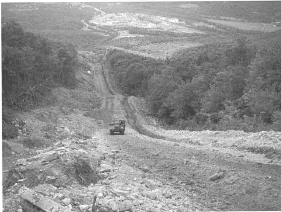
Figure 6. Example of construction road with adjacent pipeline trench. Material excavated for the road is piled on uphill side of road; material excavated for the trench is piled in a berm on downhill side of trench.
